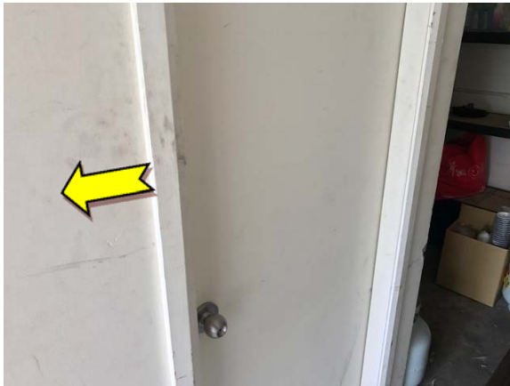
Photo 3. Interior, ground level, throughout, walls - suspected lead-containing beige upper paint system.
